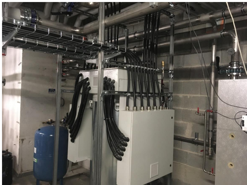
figure 2: Power to Heat with capacity of 1 MW from public swimming pool
