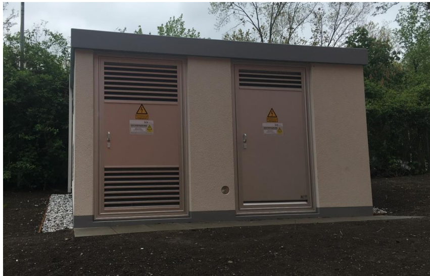
figure 3: Transformerstation for the power to heat in the public swimming pool in Amras
