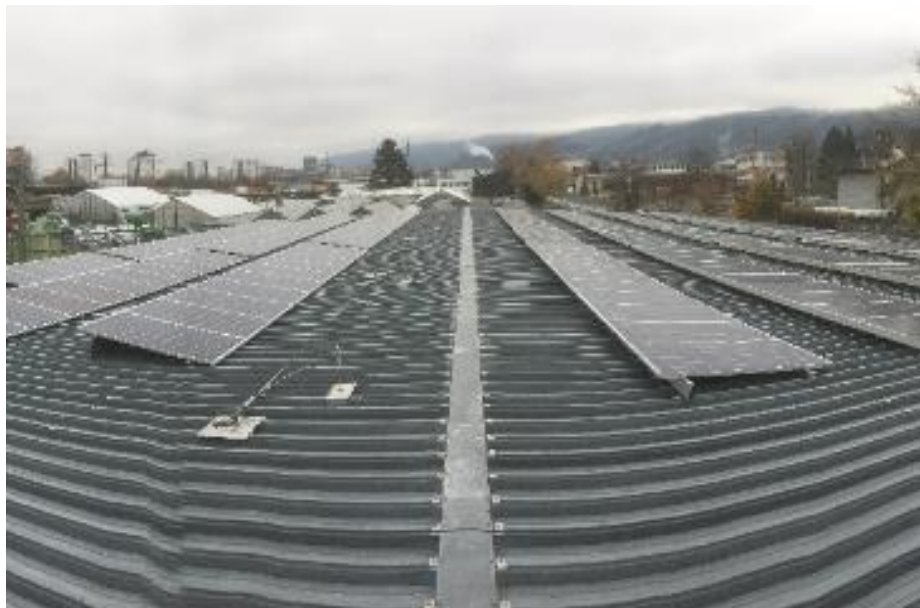
figure 8: PV plant - Trientlgasse
