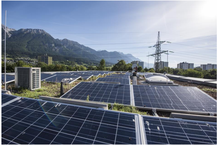
figure 7: PV plant -Recycling Center - Rossaugasse 4
