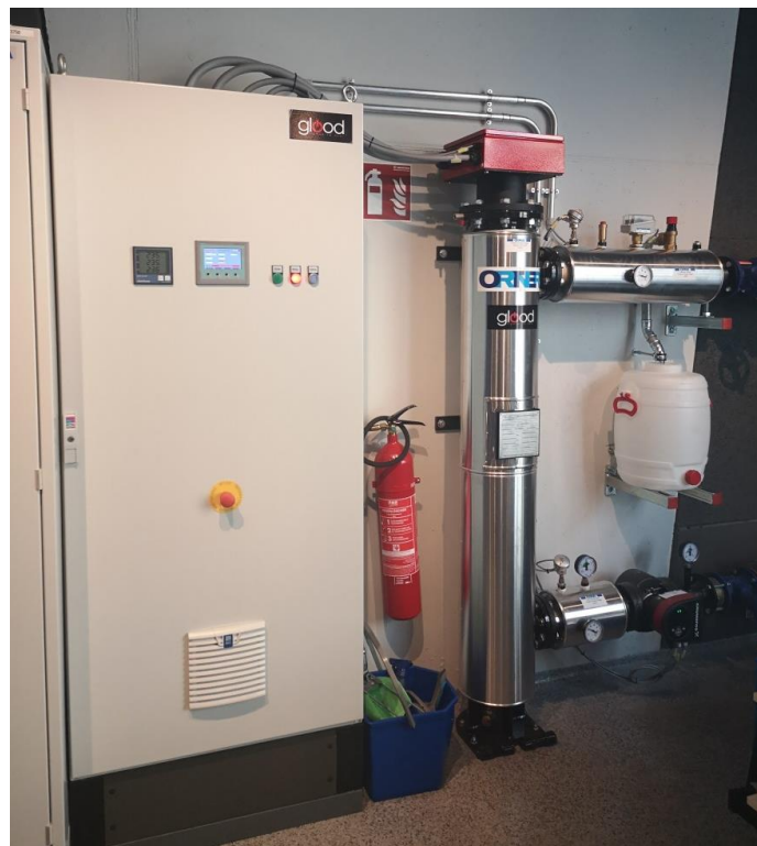
figure 4: Power-to-heat system in the IKB-Smart-District
