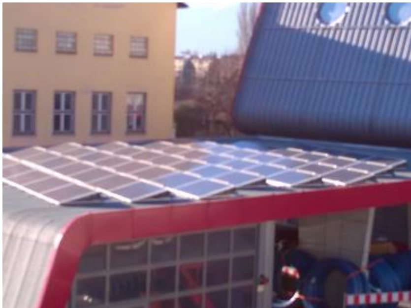
figure 6: PV plant Showroom - Langer Weg 32
