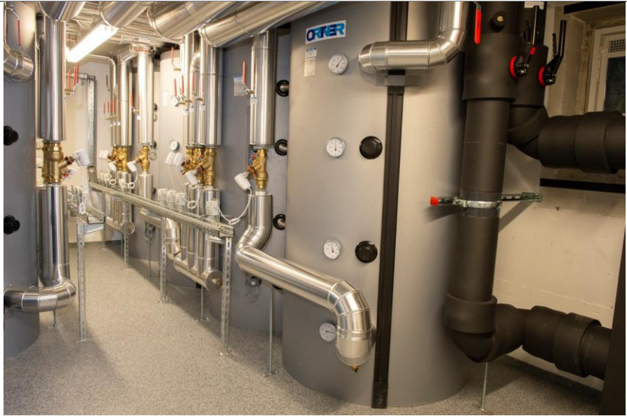
figure 3: Heat storage tank cascade – 6 x 1,500 litres
