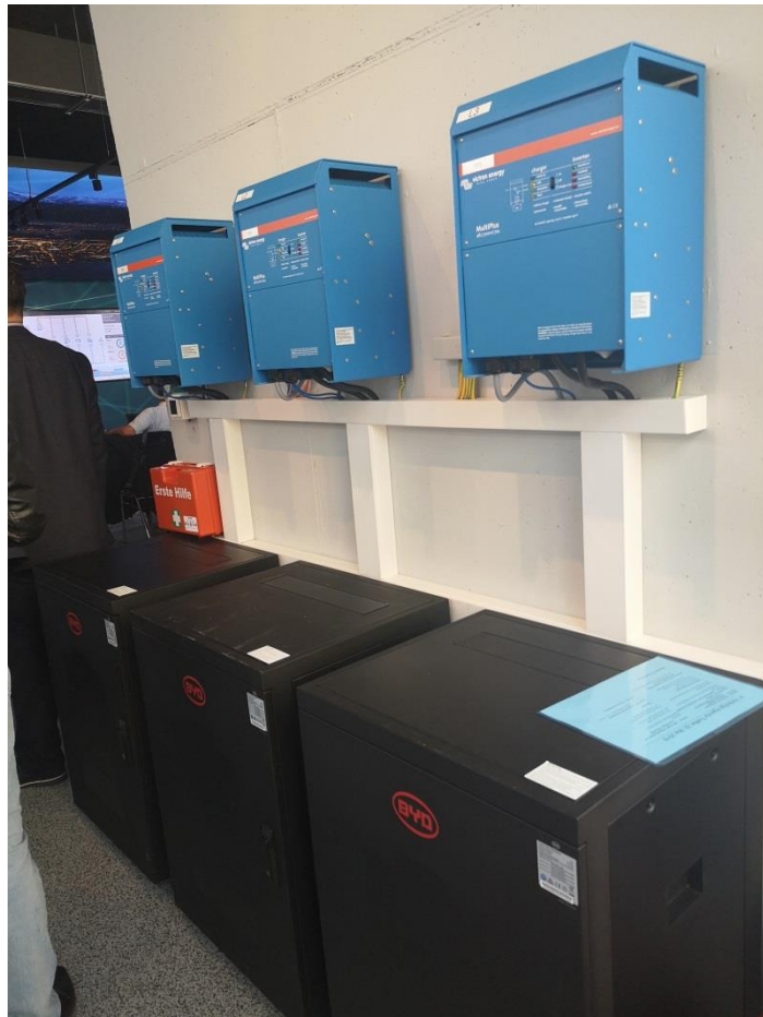
figure 9: Battery storage – Langer Weg 32
