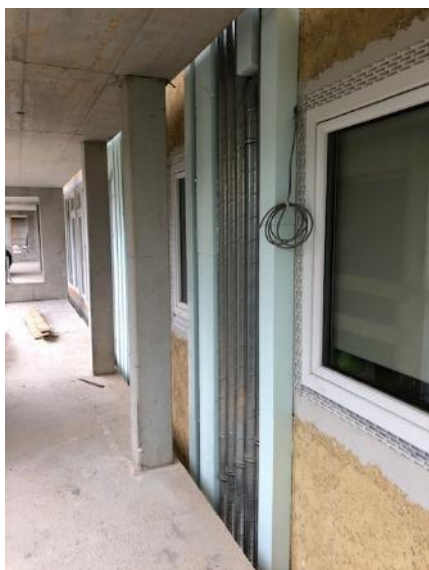
FIGURE 5: STRANDS OF VENTILATION DUCTS
