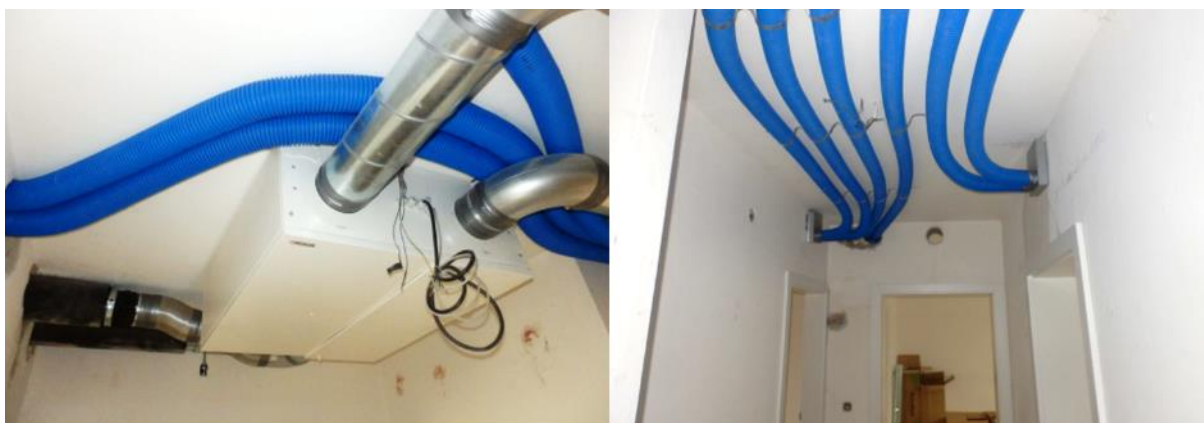
FIGURE 15: IN 40 – MOUNTING OF DECENTRAL VENTILATION UNITS AND DISTRIBUTION SYSTEM WITHIN THE APARTMENTS
