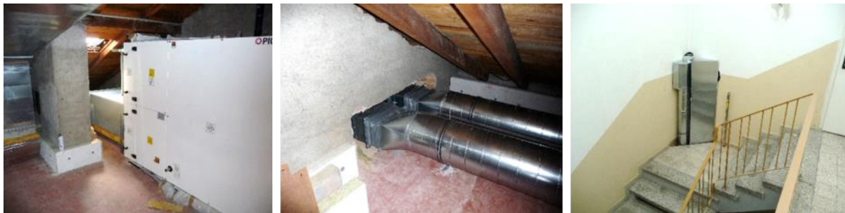
FIGURE 50: CENTRAL VENTILATION UNIT (LEFT), PIPES PENETRATING THE ROOF SKIN (MIDDLE), CENTRAL VENTILATION DISTRIBUTION (RIGHT)
