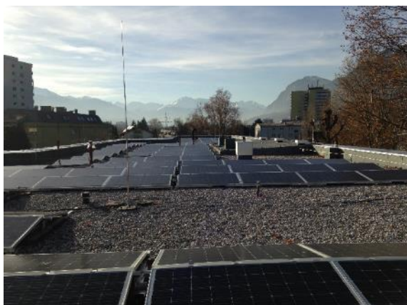
FIGURE 11: VS NEUARZL – PV POWER PLANT
