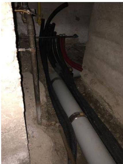
FIGURE 3: SCHUBERT-MOZARTBLOCK – VENTILATION DUCT IN THE BASEMENT
