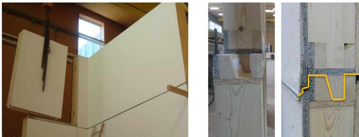
FIGURE 44: SAMPLE OF E.T. FAÇADE SYSTEM (LEFT) AND HORIZONTAL JOINT DETAIL (RIGHT) [4] © BADERGRUBER, T.; LE LEVÉ, C.
