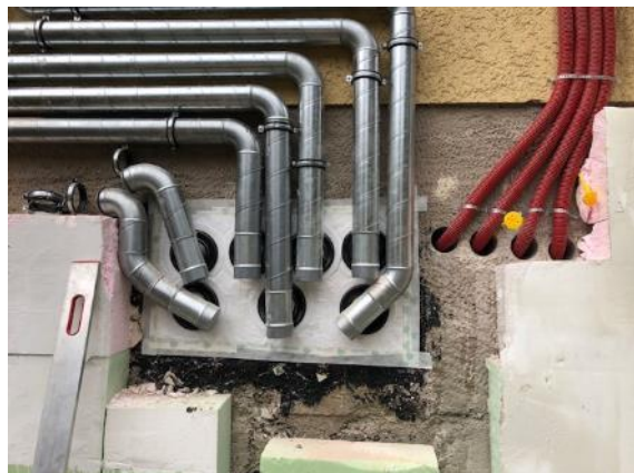
FIGURE 4: SCHUBERT-MOZARTBLOCK – MAIN DISTRIBUTION VENTILATION DUCT, ELECTRICITY AND SINFONIA MEASUREMENT TECHNOLOGY
